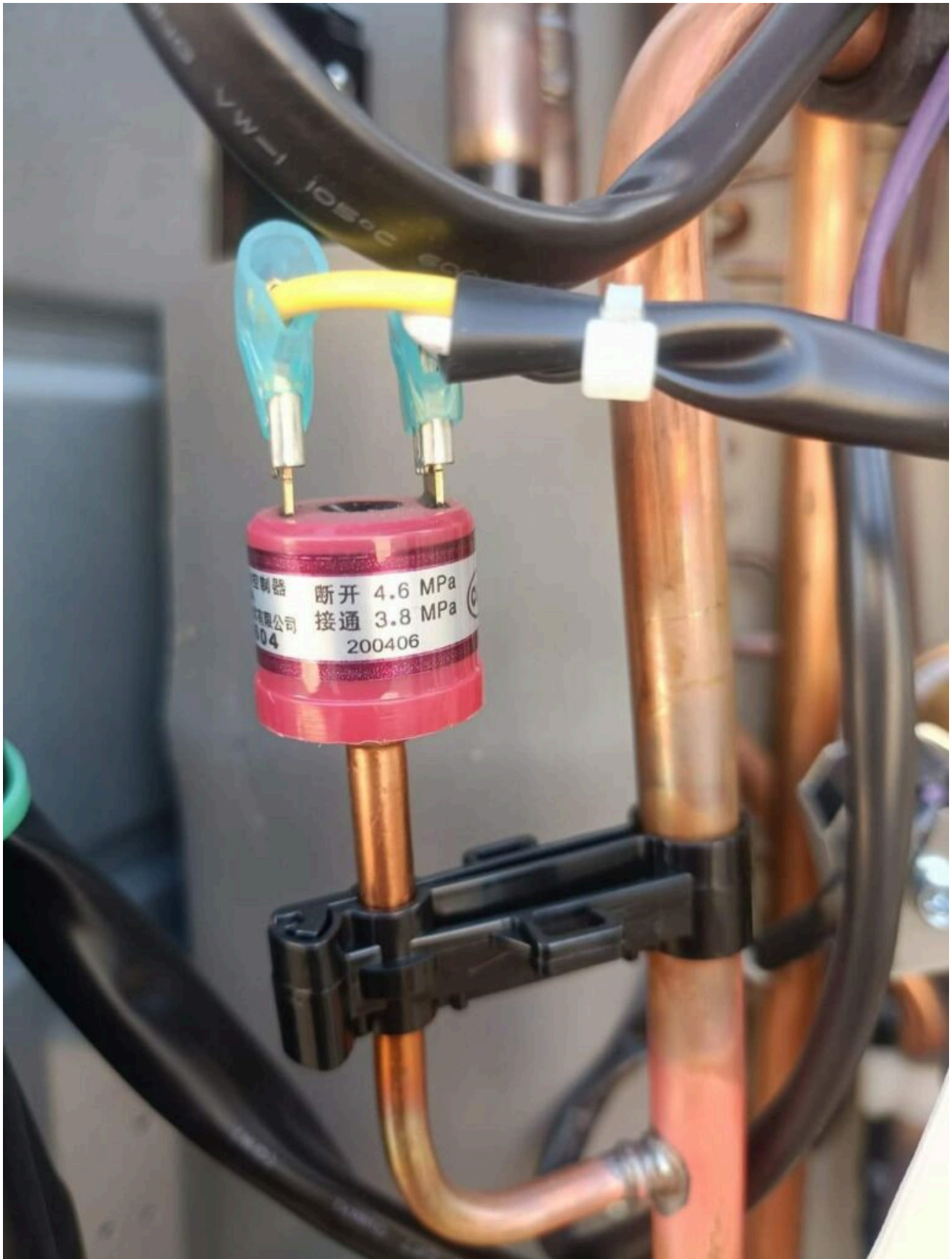
low-pressure cut-off switch
