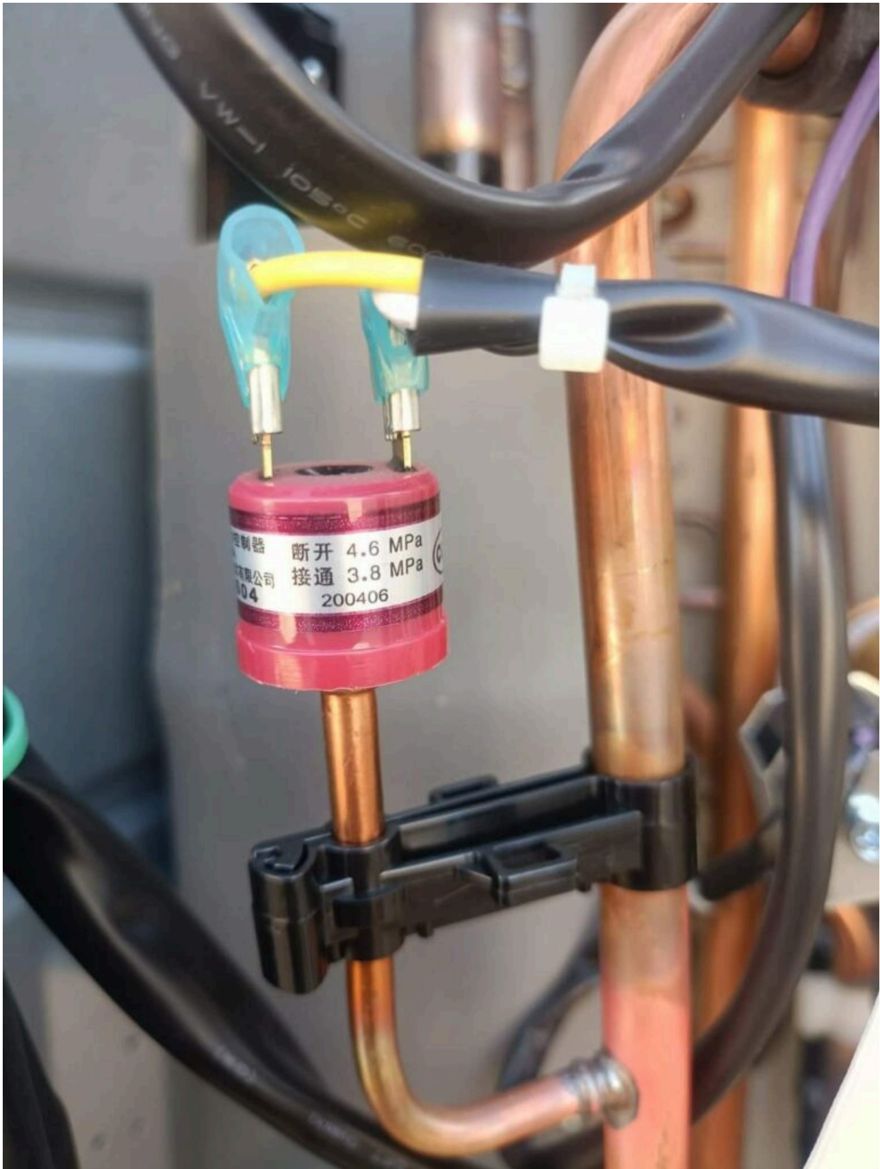
low-pressure cut-off switch
