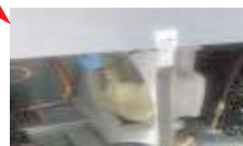
2. Check whether the C-FAN is operating
