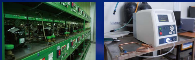
System performance equipment
